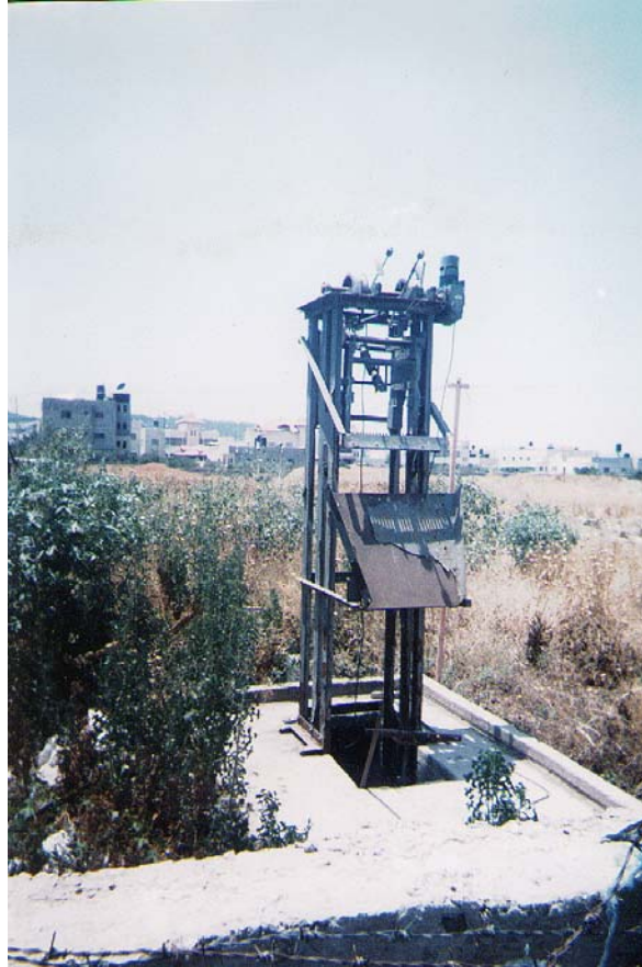
Bar Screen Unit at Jenin WWTP
