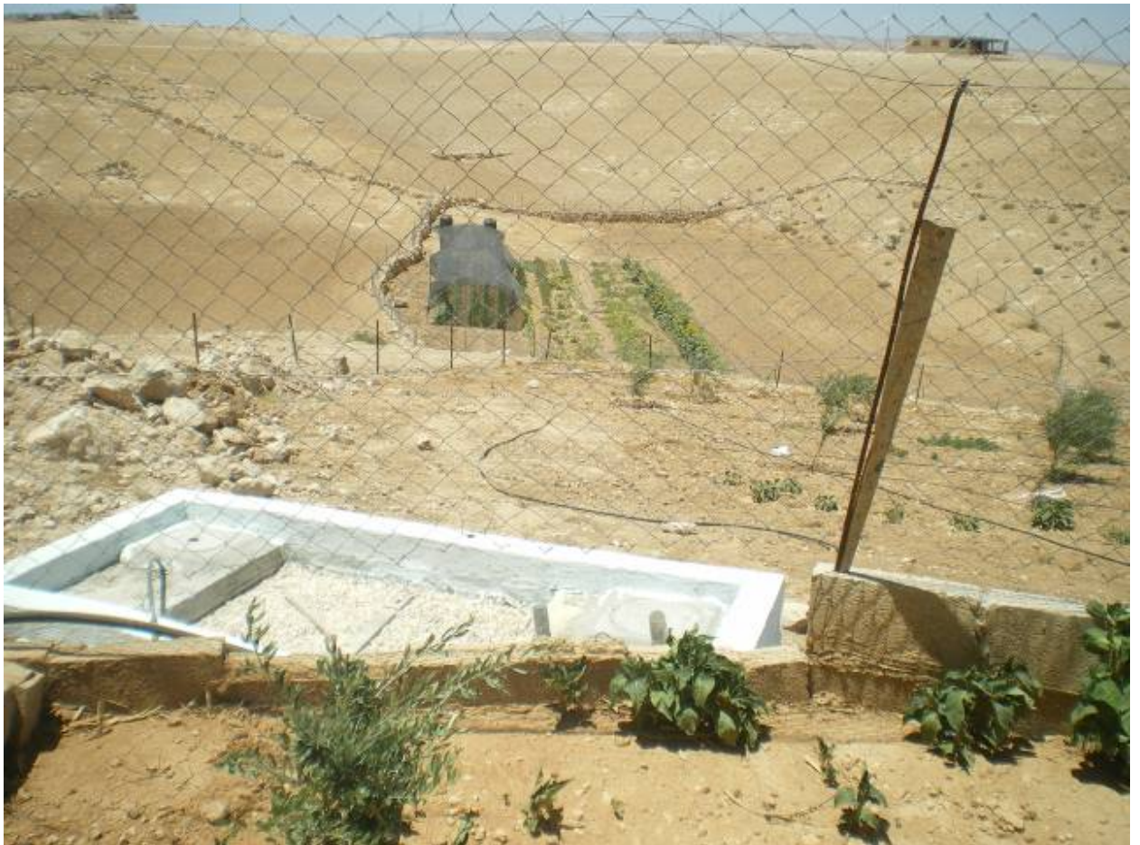
Photo (11), GWWT and Reuse System Az Zuweidin.
