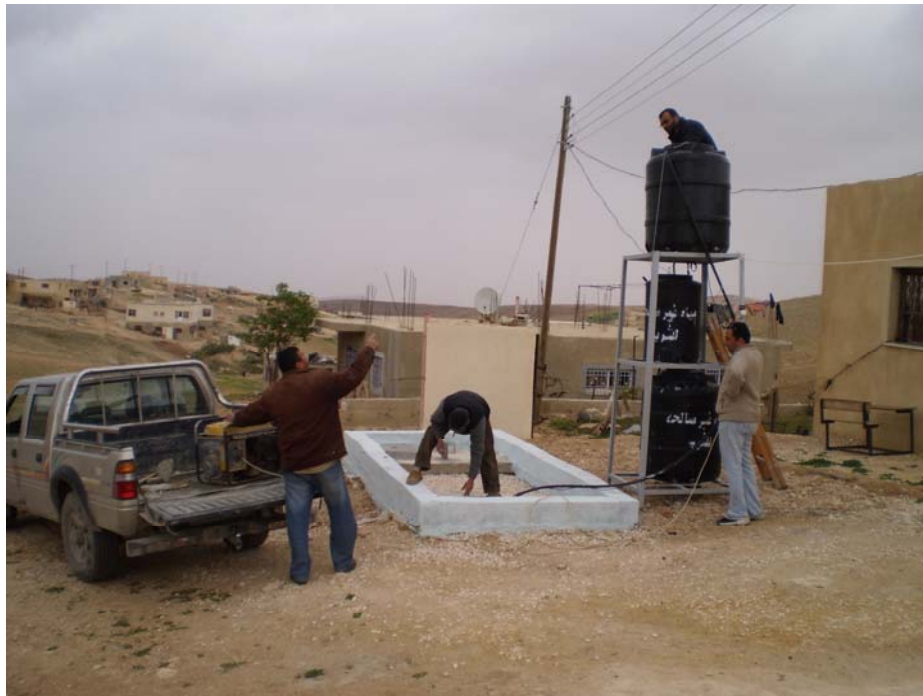
Photo (6), GWWT unit and Home garden at Az Zuweidin.
